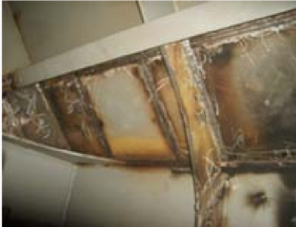
Fig.1 H1053 coating damage condition (after erection of the entire tank)
