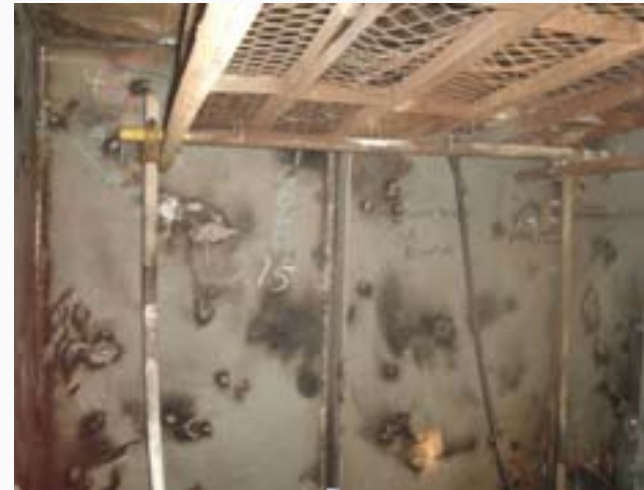
Fig.2 H1053 coating damage condition (man-made damage)
