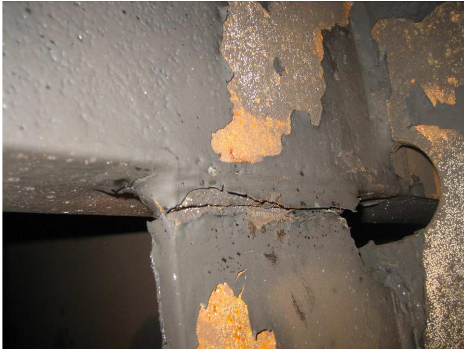
Fig.1 Discovery - The Fracture When Cleaned 20 identical cracks were found in 4Port and 21 were found in 4Stbd.
