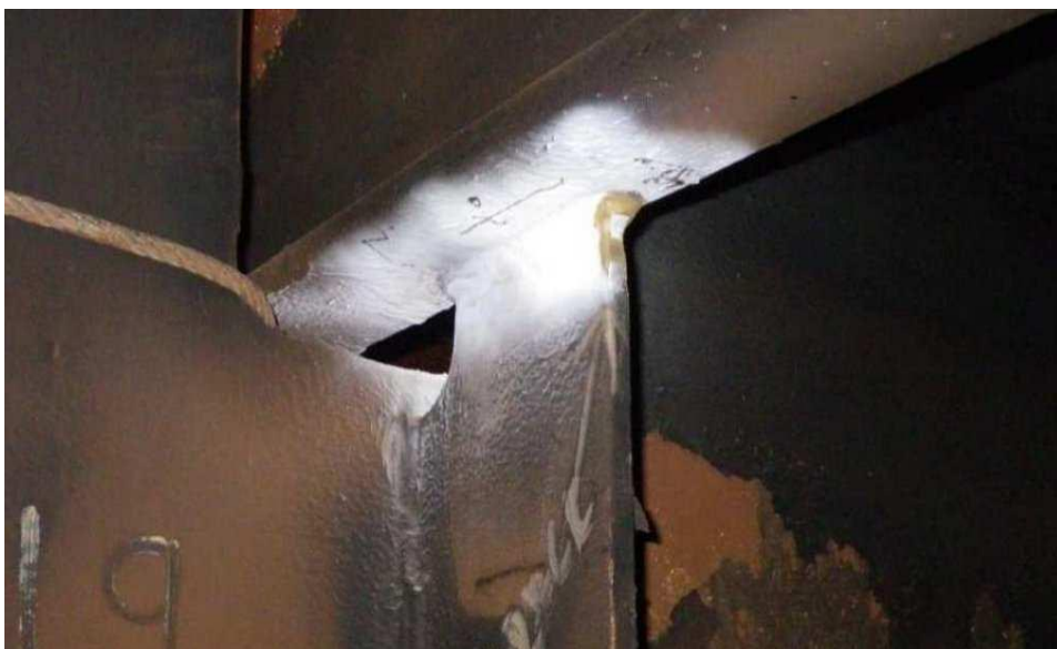
Fig.7 A Suspect Connection - The Weld
