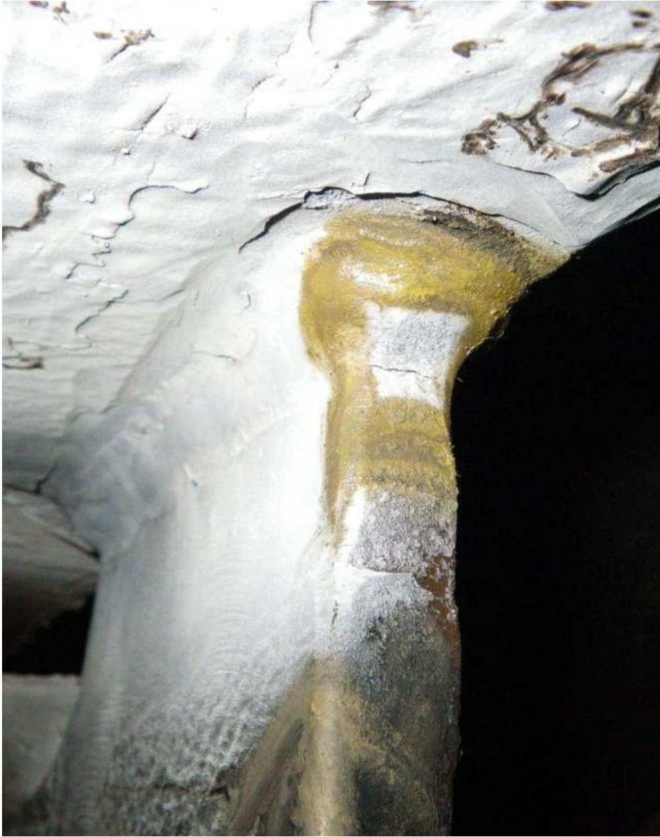
Fig.8 The Fracture - MPI Crack in the Weld Parallel to Deck
